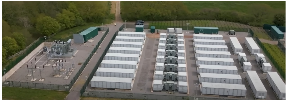
Example of 200 MWh Battery Storage
